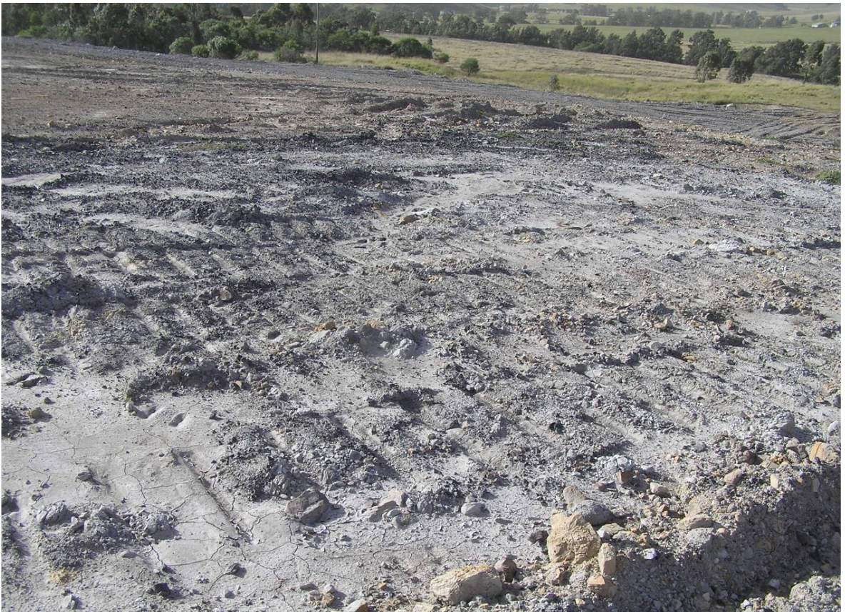
Plate 22. Antienne East – Hebden Slot. Final contouring completed. Develop and implement rehabilitation strategy.
