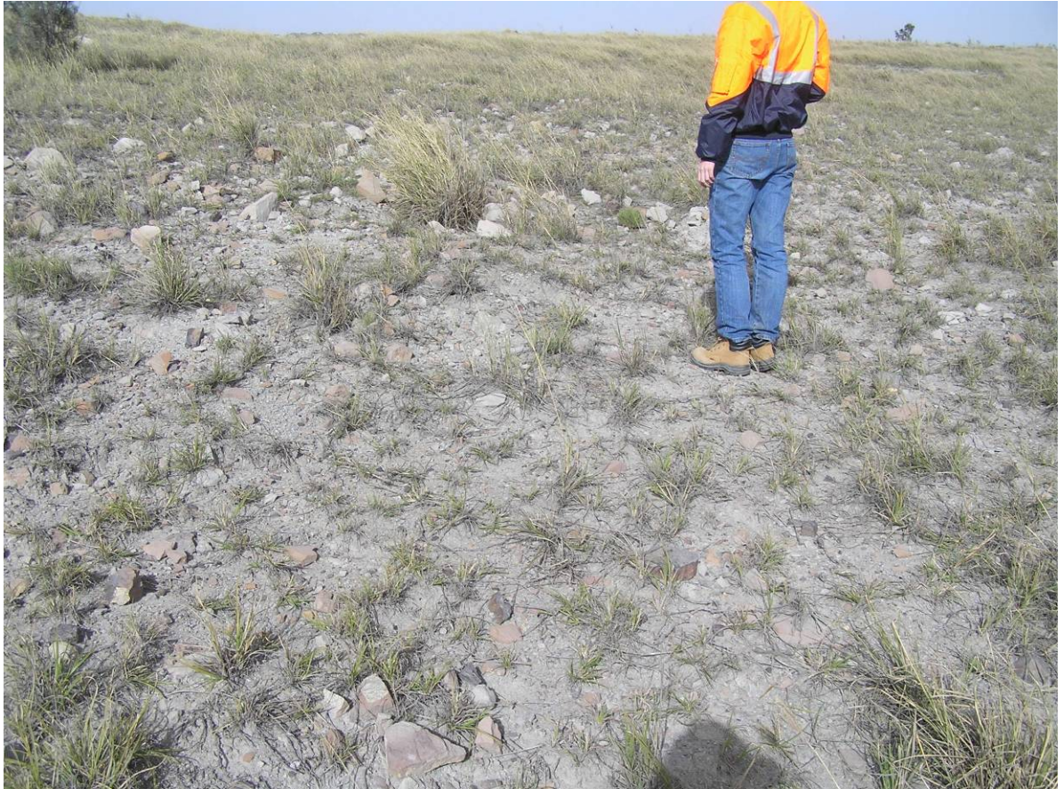
Plate 3. Lakeside Drive. Rip and reseed bare (failed) areas.
