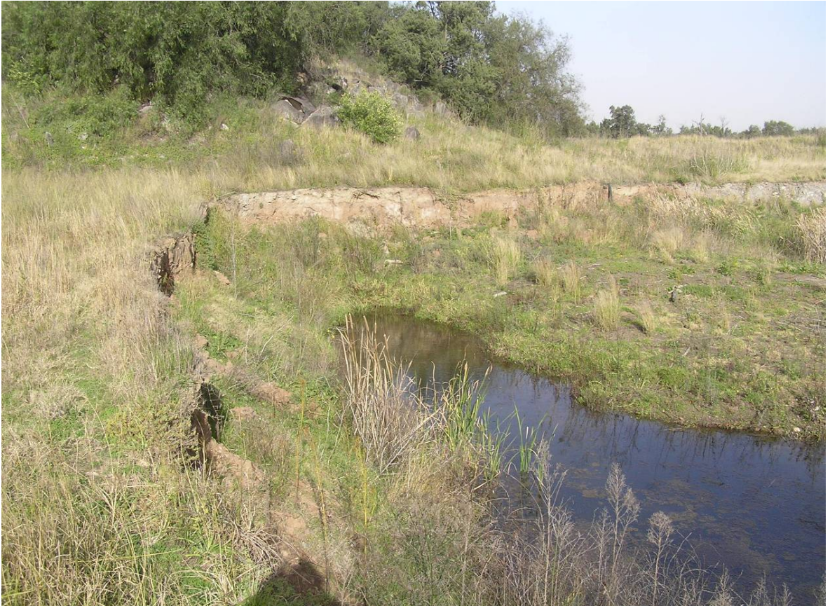
Plate 21. Antienne East. Collapsed dam wall and road. A safety hazard. Repair and re-establish.
