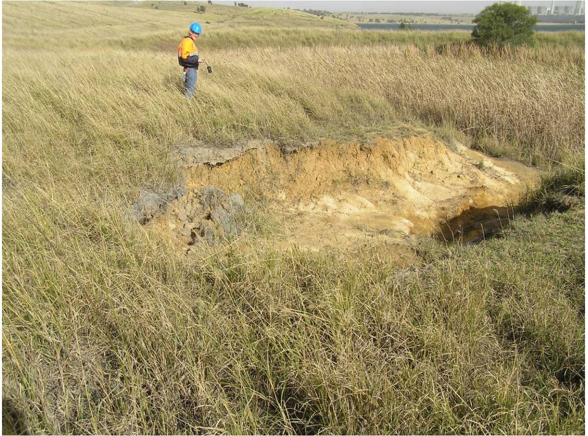
Plate 7. Lakeside Drive. Eroded entry into sediment dam needs repair. Good macrophyte development in dam.
