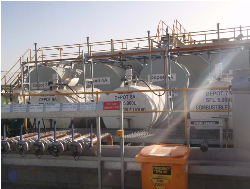
Plate 3 Liddell hydrocarbon storage areas and emergency spill kit
