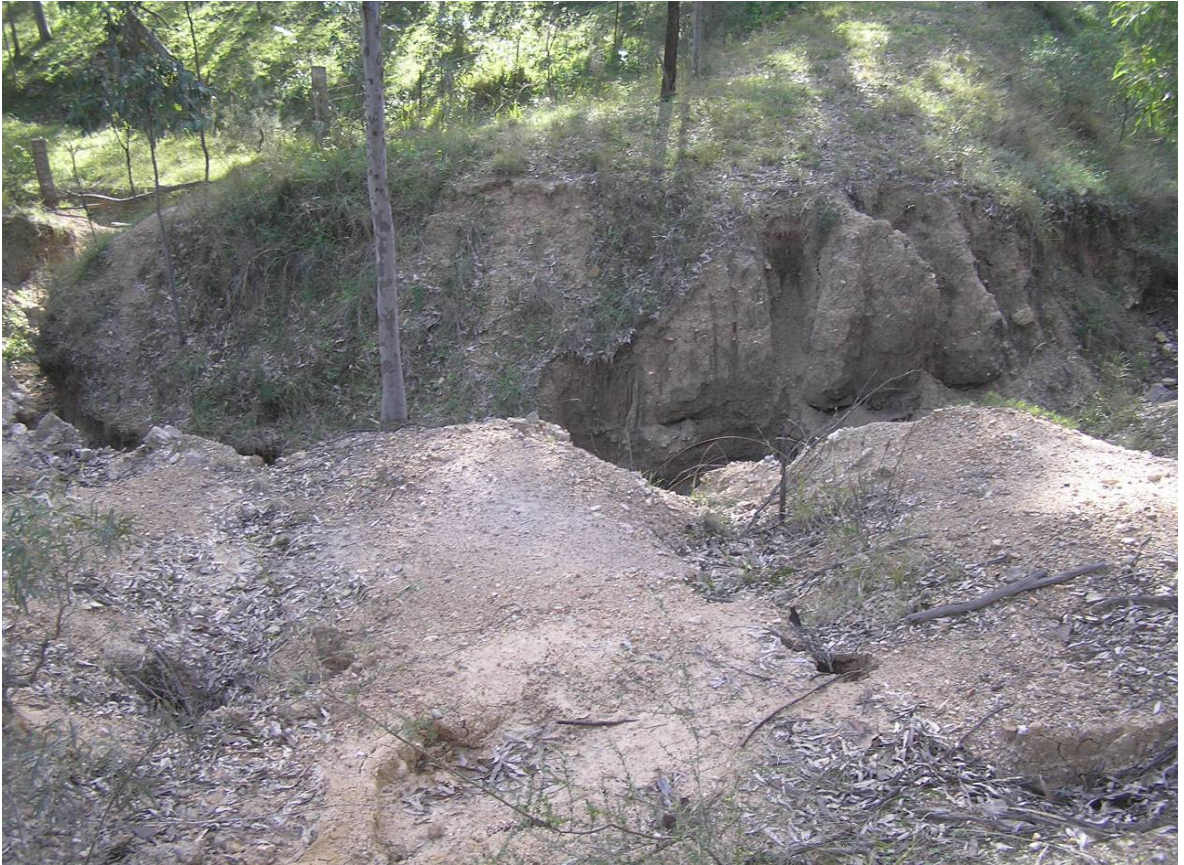
Plate 25. Mountain Block. Repair failed sediment dam walls (several dams in this vicinity).
