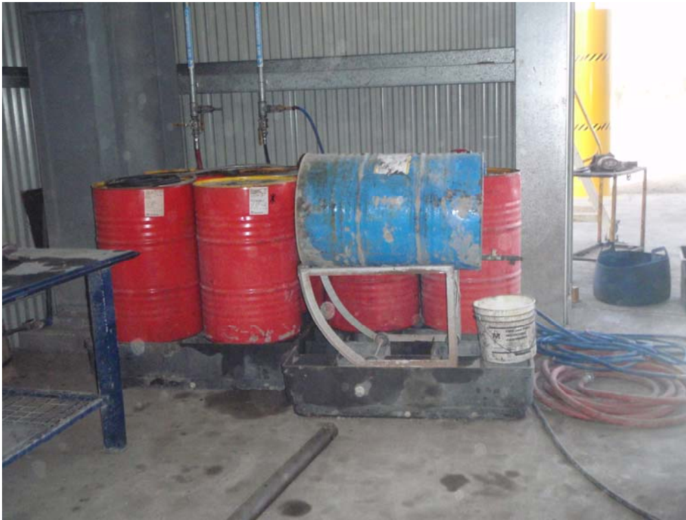
Plate 1 Bunded hydrocarbon facility in the Liddell workshop
