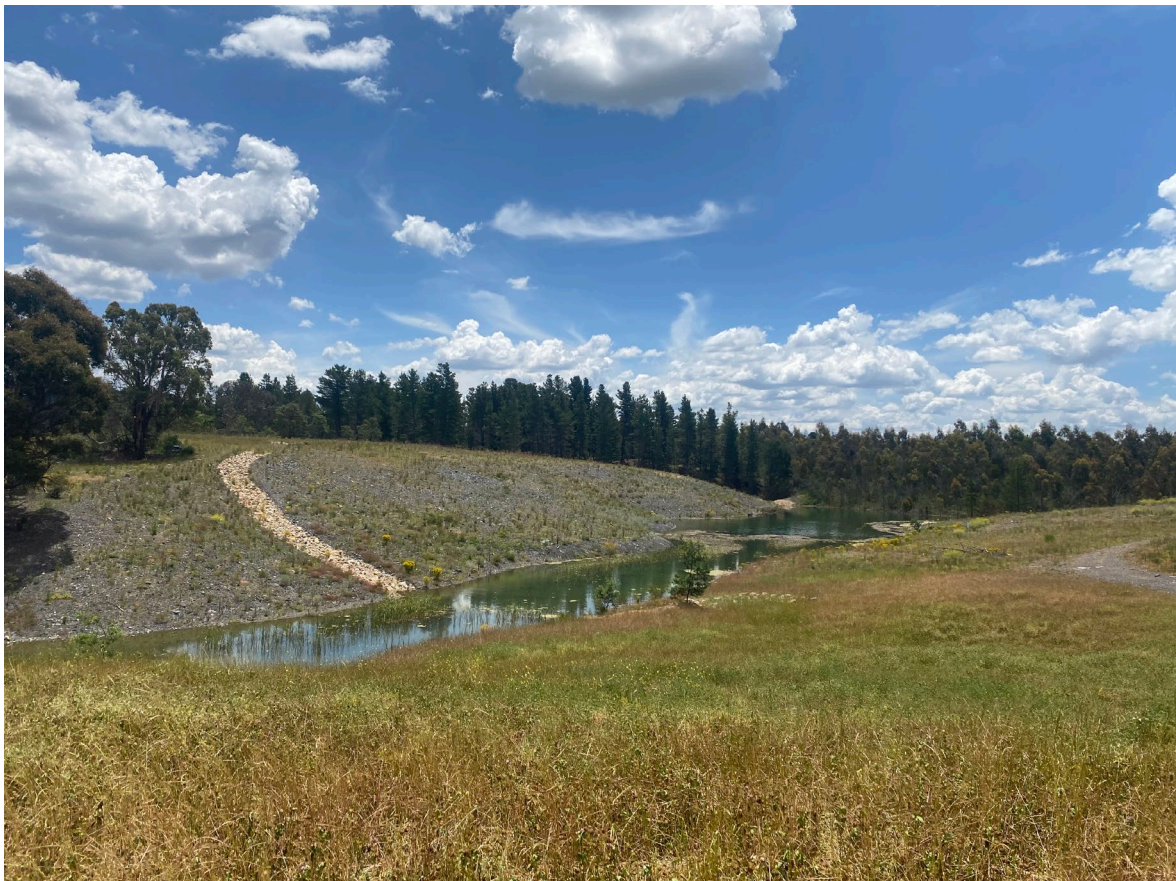
Photo 12 – Further rehabilitation required on steeper sections where shale is exposed.
