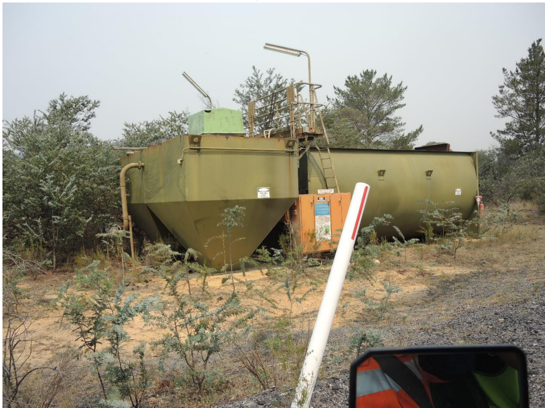
Plate 14 On-site Sewage Treatment Plant
