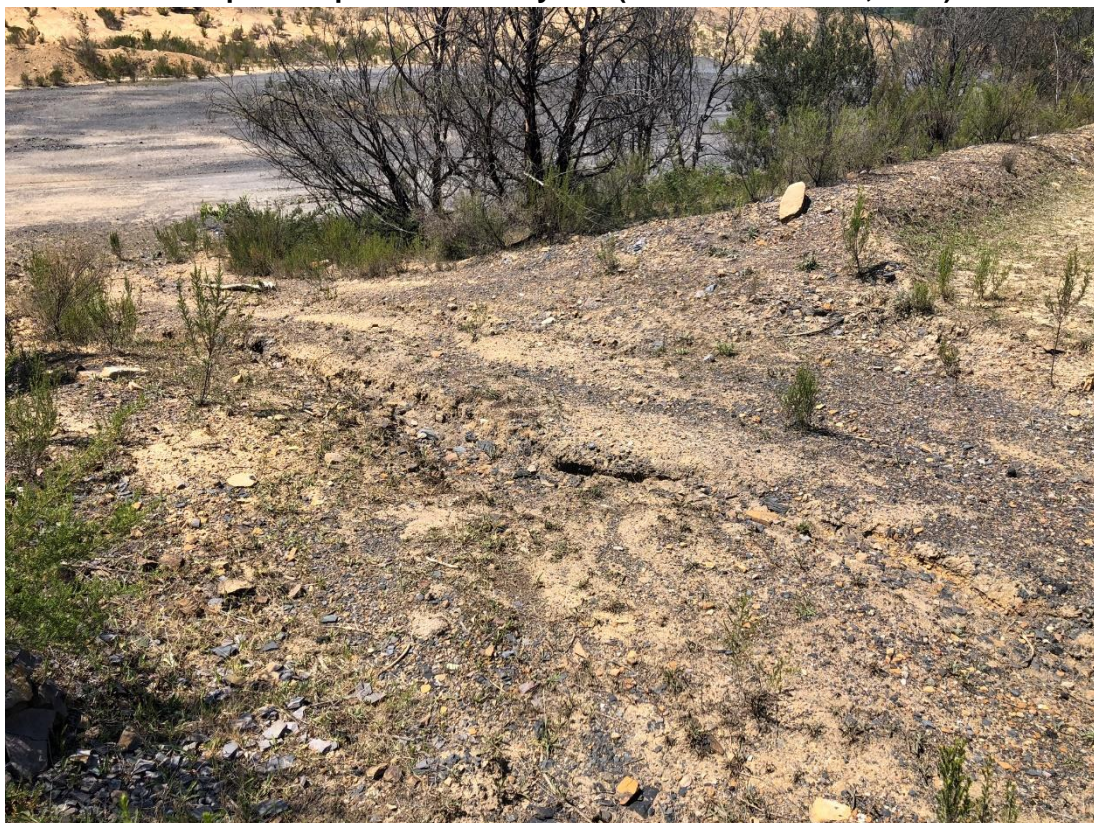
Plate 4 Contour drainage bank breached by access track on Thistle Hill, requires repair (Source: Minesoils, 2020)
