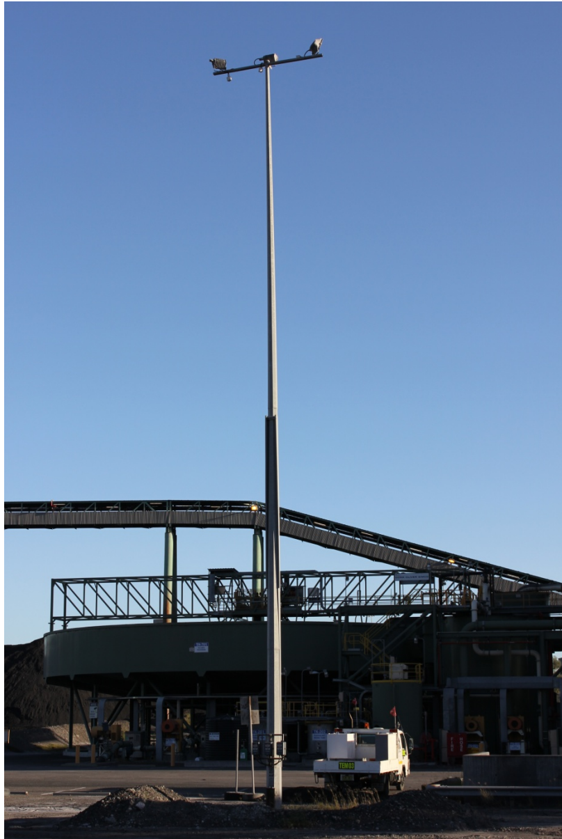
Internal site 3 (day) light tower at CHPP
