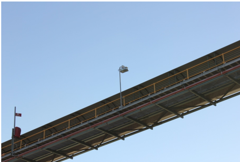
Internal site 3 (day) lighting on conveyor
