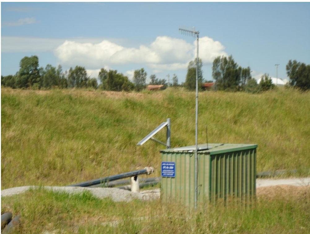
Plate 14 Existing EPL Discharge Point
