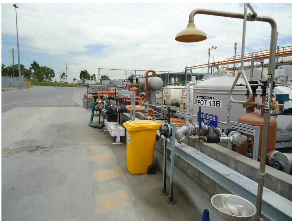
Plate 4 Bulk Fuel Storage Fill Point
