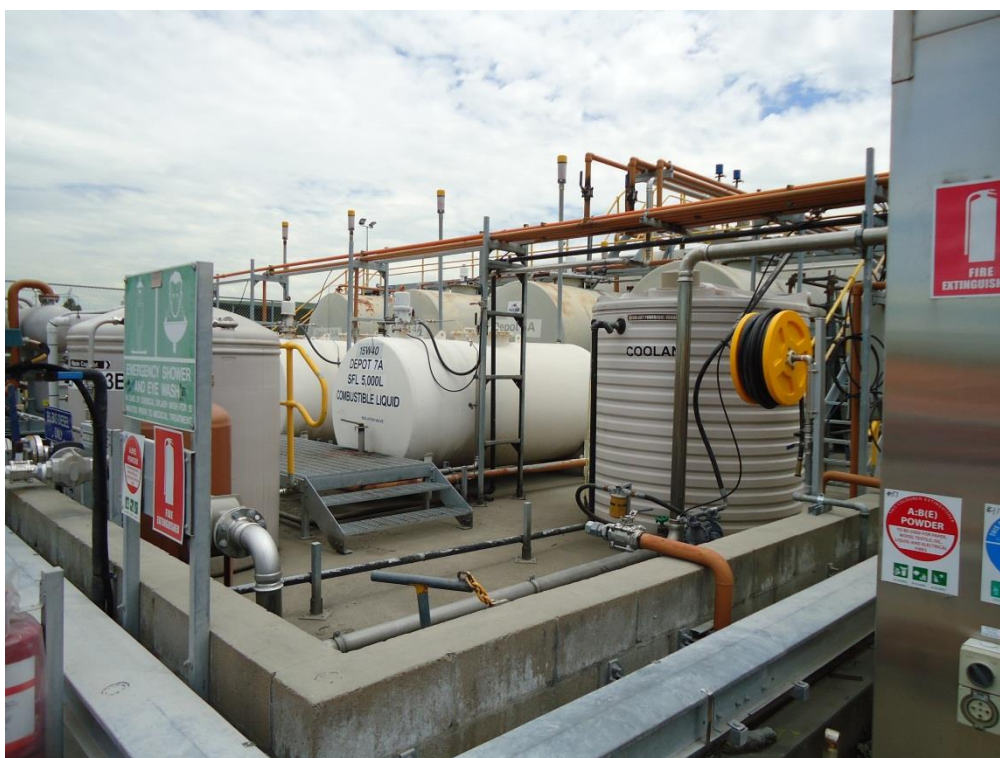
Plate 3 Bulk Fuel Storage Tank Bunding
