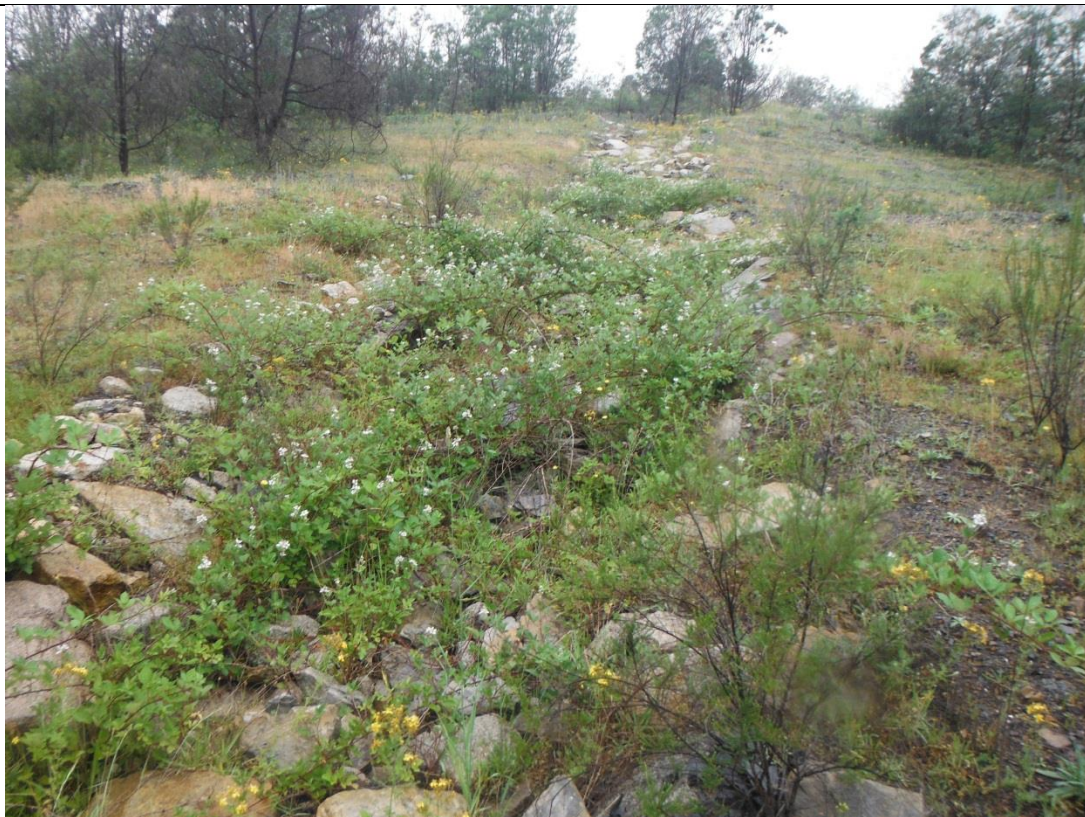
Photo 10 – Drop structure is well designed and functional but is covered by Blackberry
