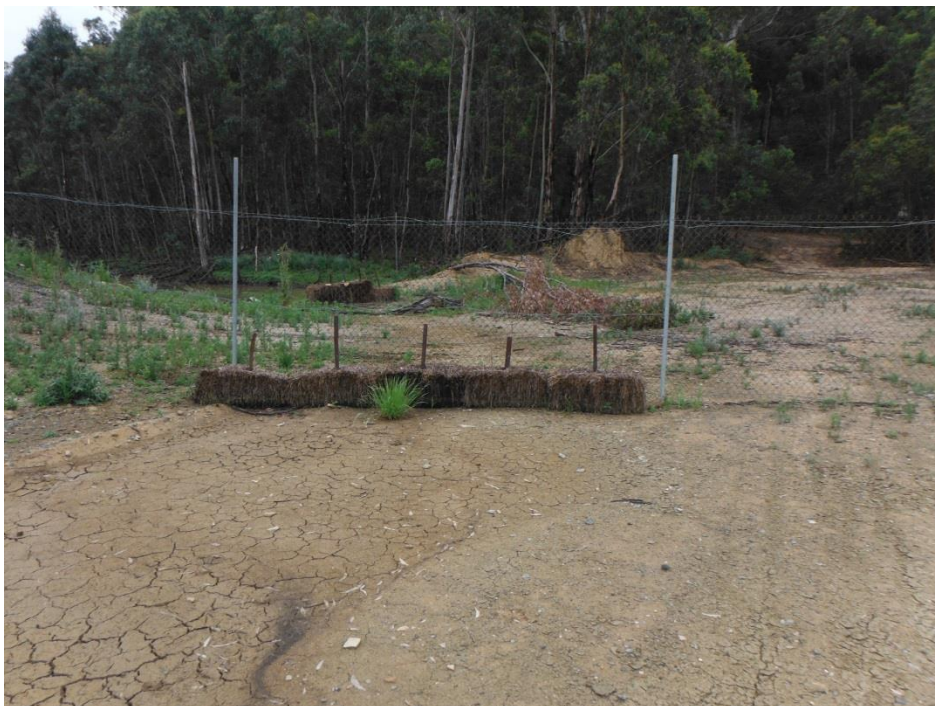
Photo 2 – Additional water management work required around REA 5 rehabilitation
